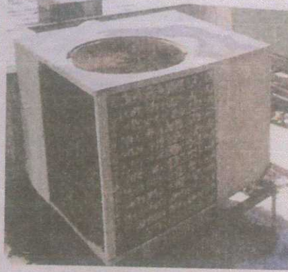
Summer air-conditioning system.
